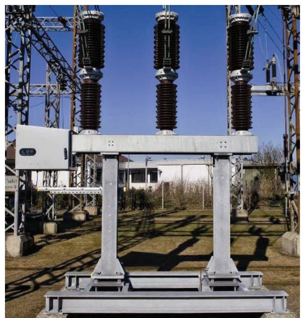
Figure 8 : Photograph of the pilot circuit breaker at utility C
